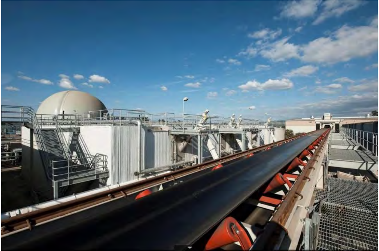
Figure 17: High Solids AD Plant, Perris, CA
