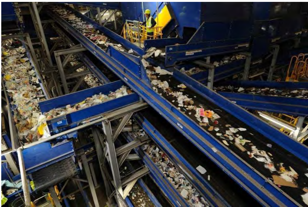
Figure 24: Newby Island Resource Recovery Park, California
