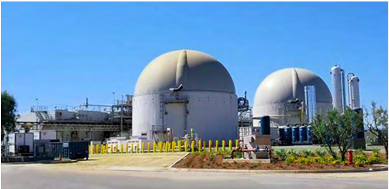
Figure 18: Vertical High Solids AD Plant, Perris, CA
