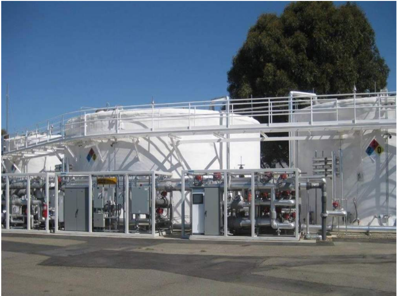
Figure 14: Low Solids AD Plant, Sacramento, CA
