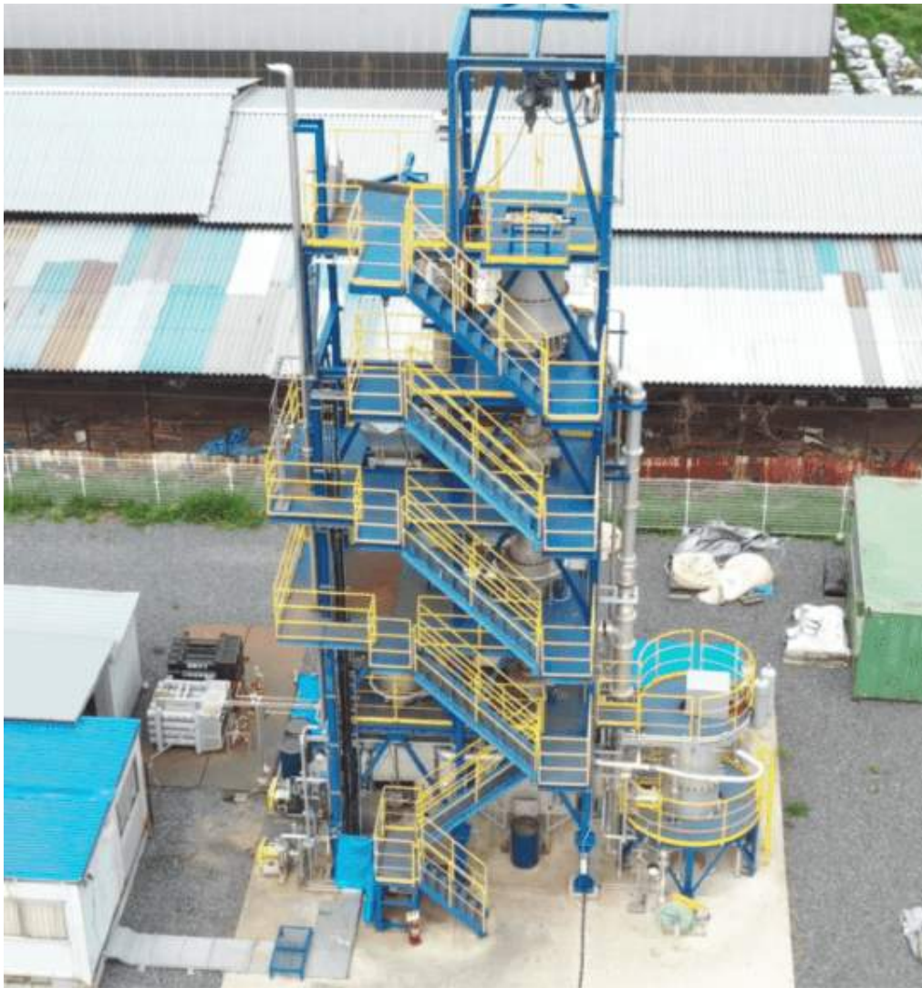
Figure 7: Ways2H Pyrolysis Facility Kern County, CA
