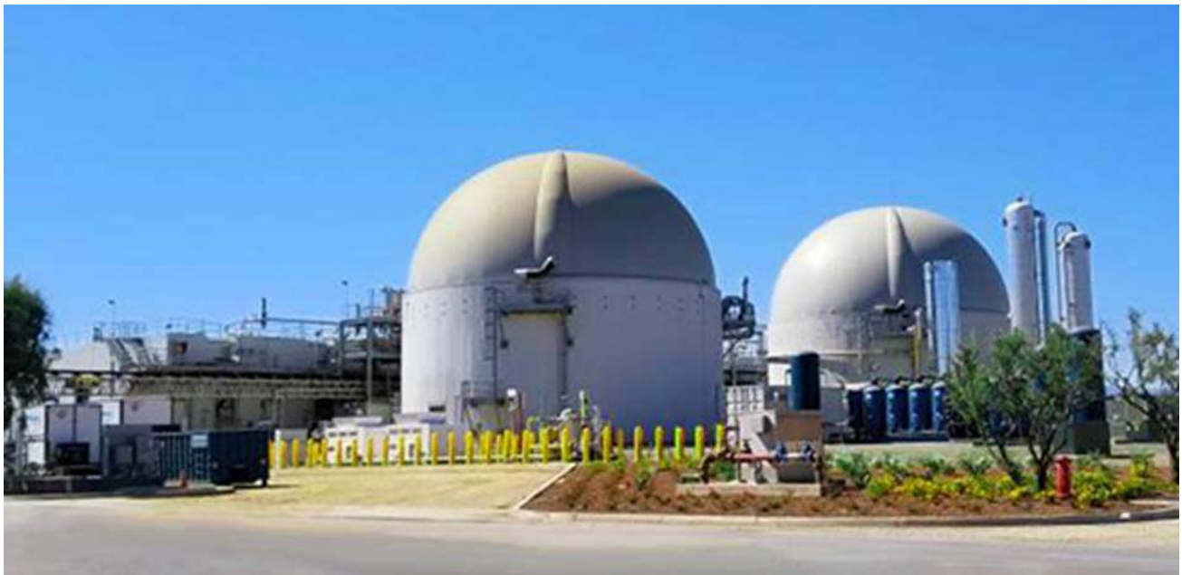
Figure 18: Vertical High Solids AD Plant, Perris, CA
