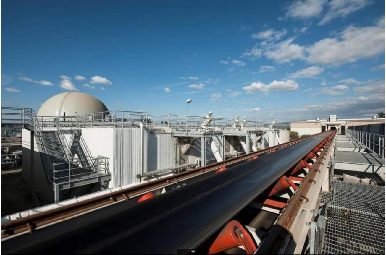
Figure 17: High Solids AD Plant, Perris, CA
