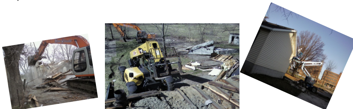
Large equipment used in the study included (l-r) excavator, skid loader with fork, and man lift.
