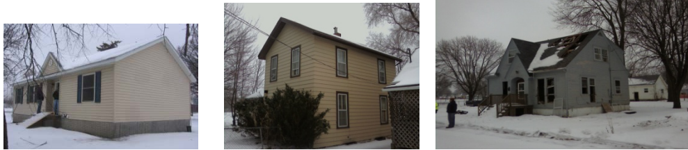
A type of hybrid deconstruction was applied to three Cedar Rapids houses that were flooded in 2008—two on the southeast side and one on the northwest side.
